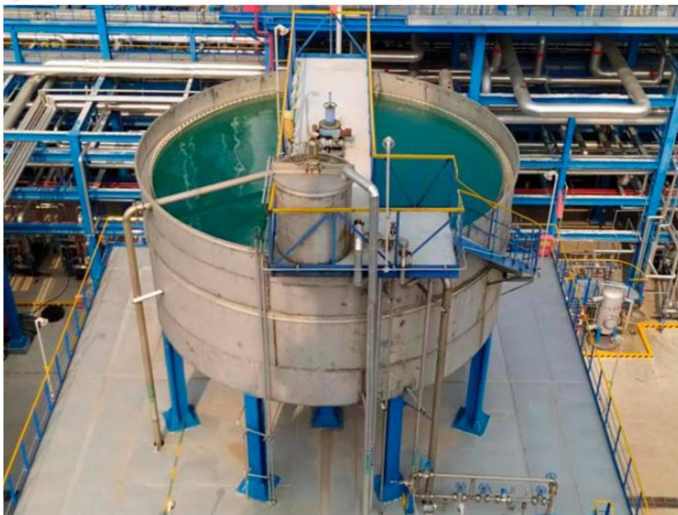
Treatment tank for wastewater from flue gas desulfurization
