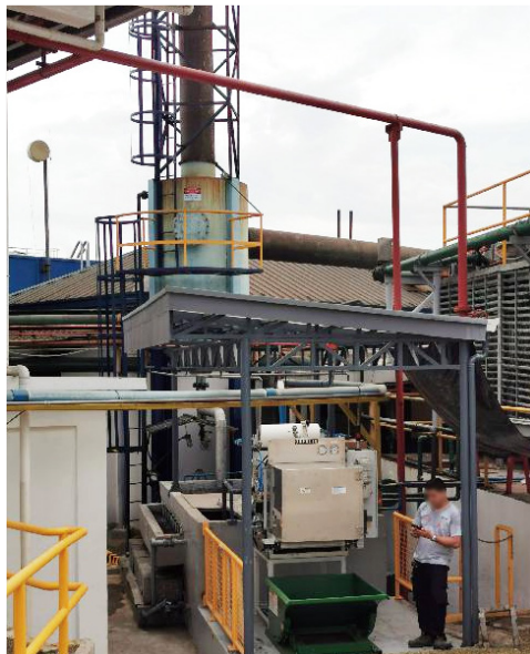
▪ Water treatment system for desulfurization units
