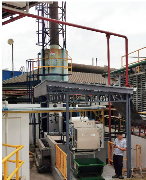
▪ Water treatment system for desulfurization units
