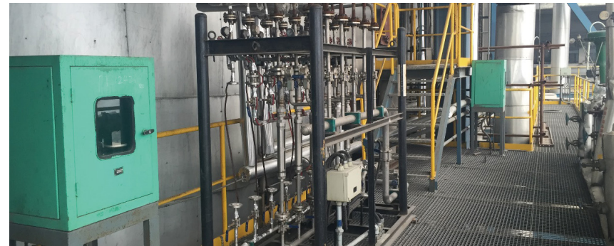
▶ 2×310 t/h Power Boiler Flue Gas Denitrification Project In a Refining Company of Sinopec
